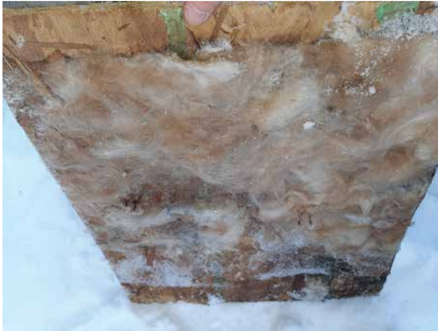
Photo 2: Wet and frozen insulation and OSB sheathing.
