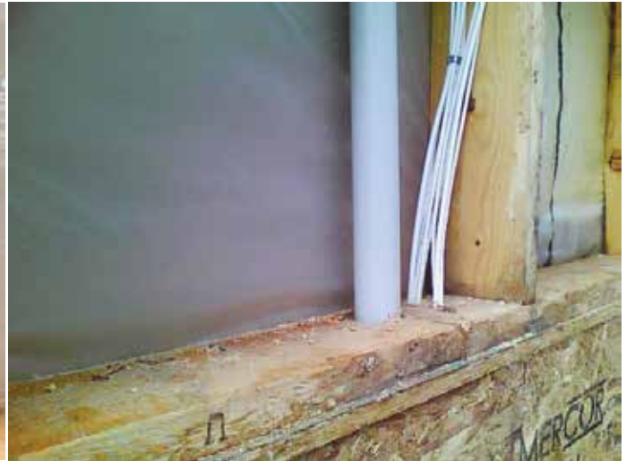
Photo 5: Typical unsealed plumbing and electrical penetrations extending through the second-floor sill plate.
