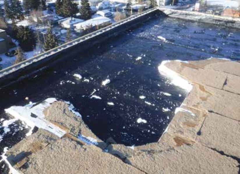
Photo 2 - Roof blown off at northwest corner of building.
