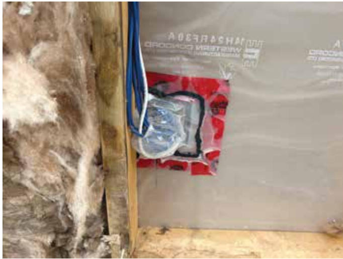
Photo 4: Unsealed cable penetrations through the polyethylene sheet.
