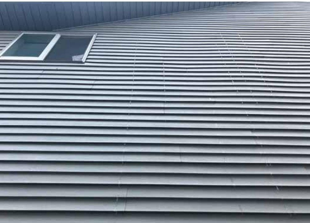
Photo 1: Water dripping from behind the siding.
