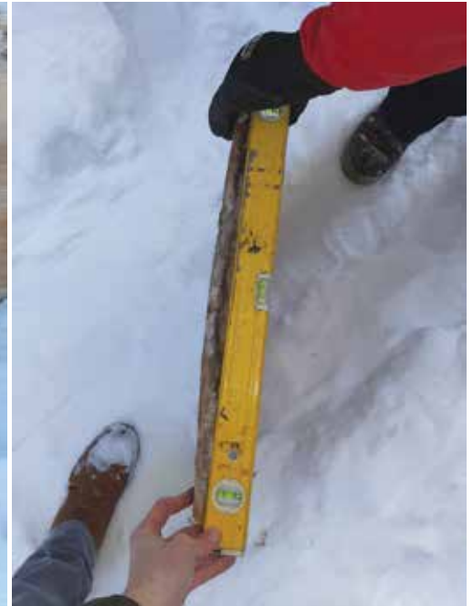
Photo 3: Bowing in the OSB sheathing.
